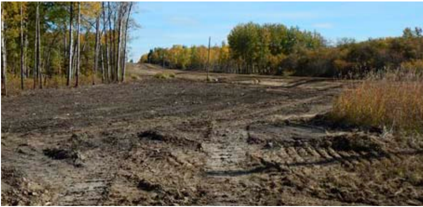
Unlawful road construction destroyed part of the Meanook National Wildlife Area in Athabasca County, Alberta, resulting in a $300,000 penalty.
